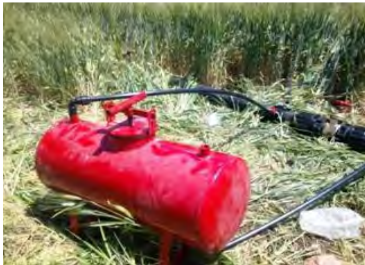
Photo 1: Views of the installation process of the drip system in the farmers' plot (top: manifold installation, middle: laterals' installation, bottom: Fertigation tank installation)
